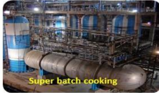
Super Batch Digesters SP. Steam Cons < by 30%
